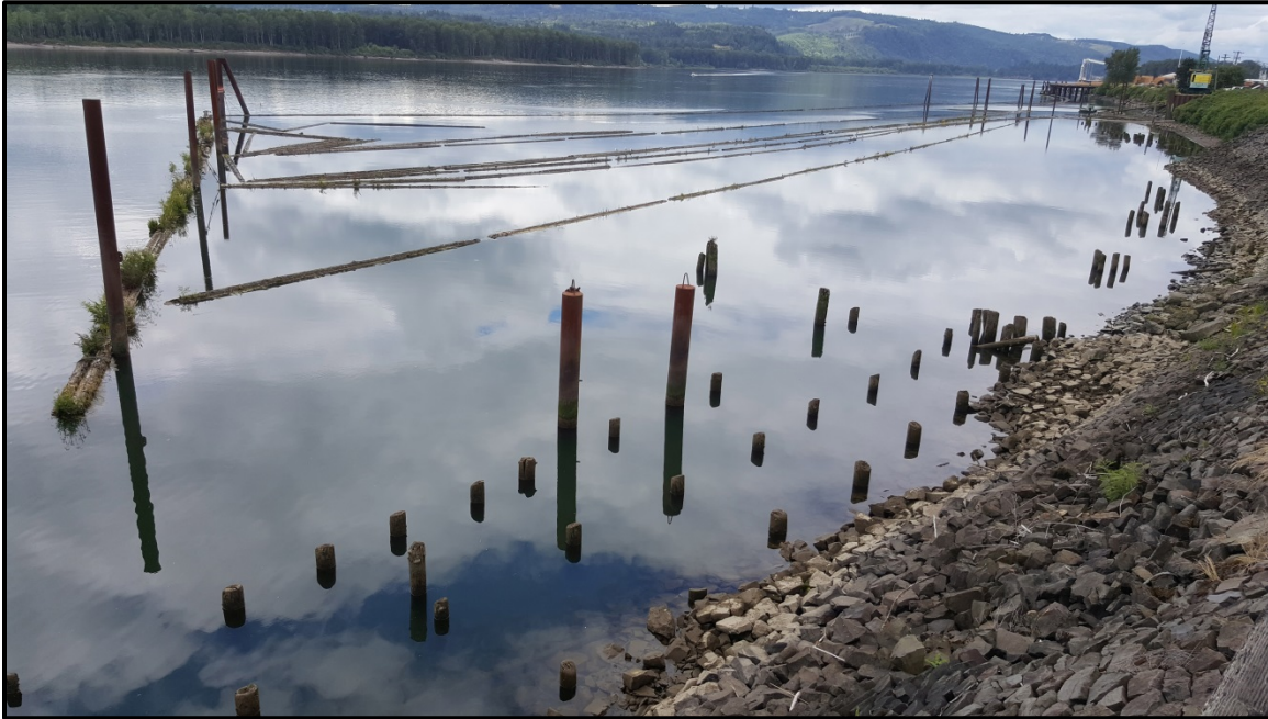
Figure 6. Northwest-facing view of the northern piles proposed for removal, with the two steel piles at photo center.
