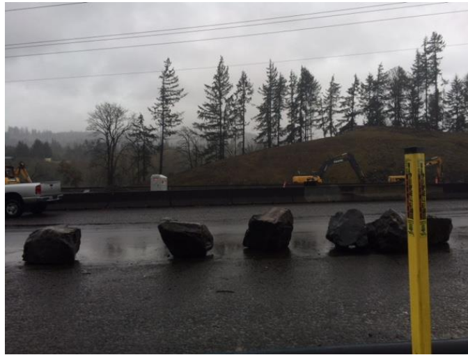
Photo 3 is taken facing east across the southern section of the proposed improvement site. This photo was taken to document the existing paved portions of the study area where some construction will occur.
