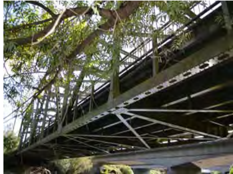
Photo 2. The west elevation of the bridge structure where piped utilities will be installed at the bottom chord. The view is towards the east.
